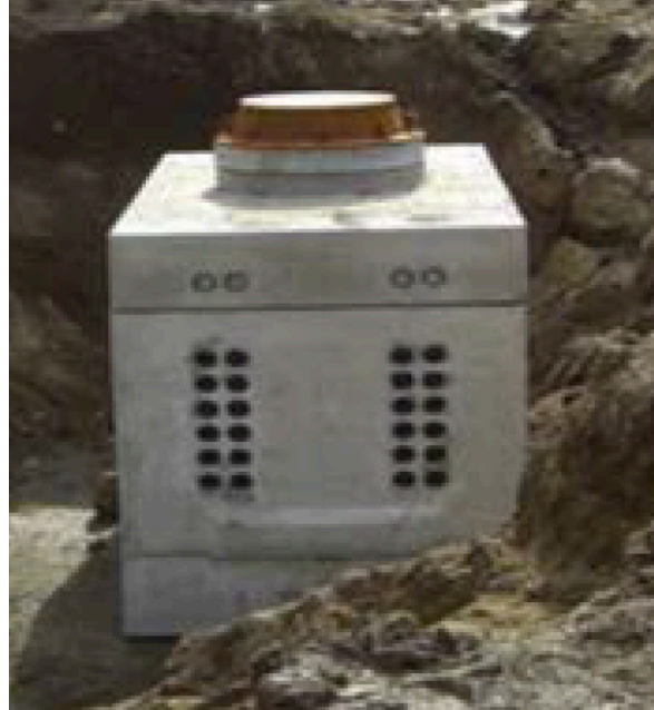
Figure 31 — Manhole for fiber patching in Virginia Beach 50
