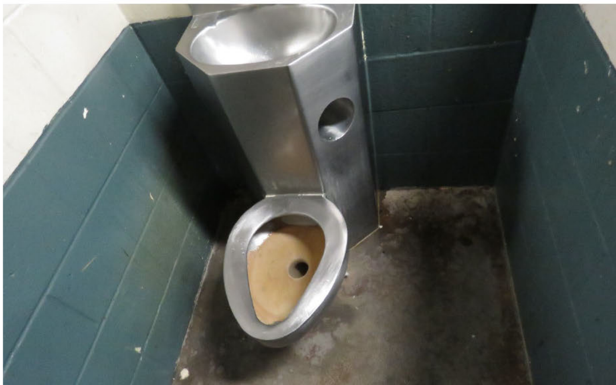
Photograph 2 – Same toilet at rear of main IRC Clinic area, looking into the bowl
